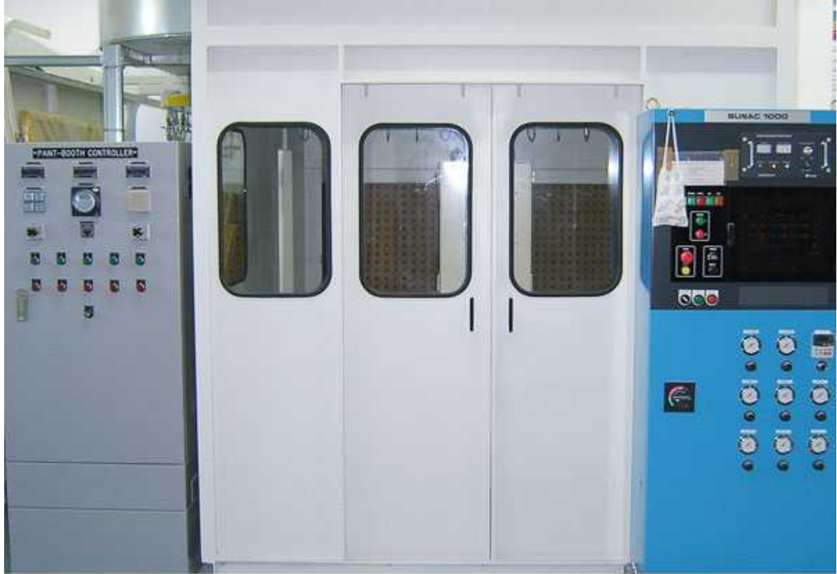
MAIN PAINT BOOTH WITH ELECTRIC CONTROLLER
